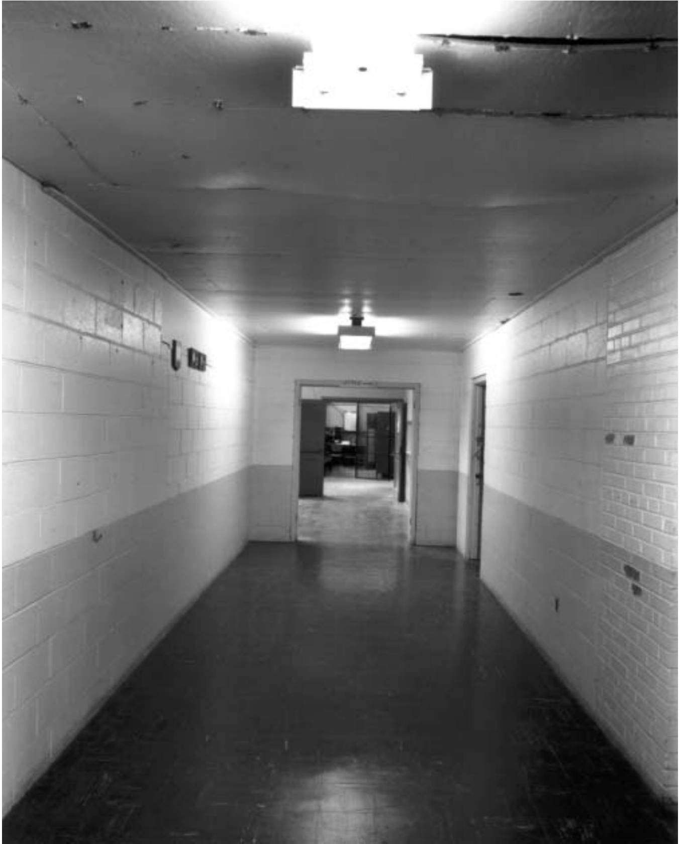
PHOTO No. 12. VIEW LOOKING SOUTH ALONG THE MAIN CORRIDOR IN THE ONE-STORY VOLUME. (SEPTEMBER 2002). PHOTOGRAPH BY TERRY RISHEL.
