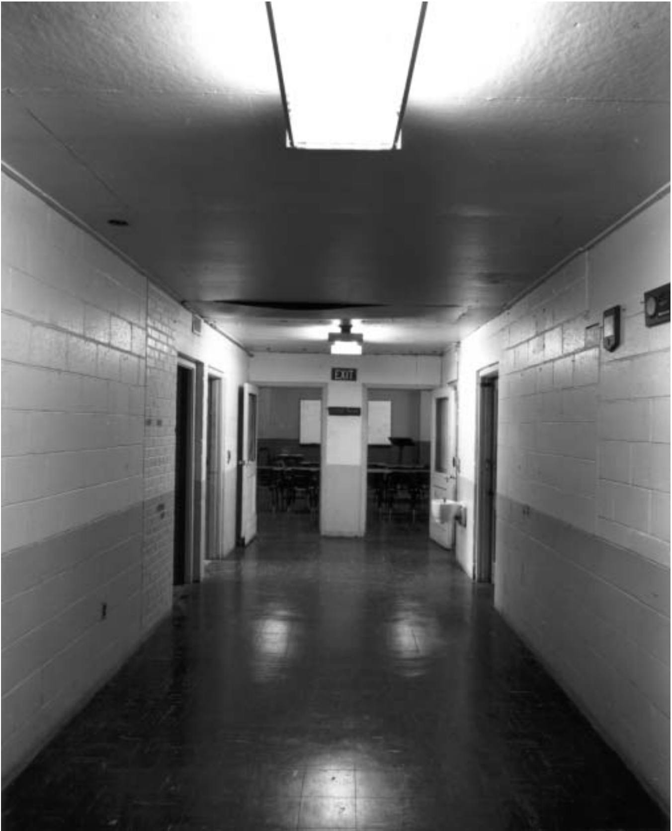
PHOTO No. 11. VIEW LOOKING NORTH ALONG THE MAIN CORRIDOR IN THE ONE-STORY VOLUME. (SEPTEMBER 2002). PHOTOGRAPH BY TERRY RISHEL.
