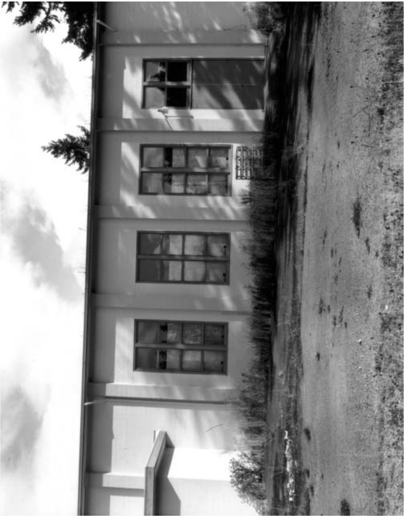
PHOTO NO. 8. VIEW OF WEST BACK OF TWO-STORY VOLUME. (SEPTEMBER 2002). PHOTOGRAPH BY TERRY RISHEL.
