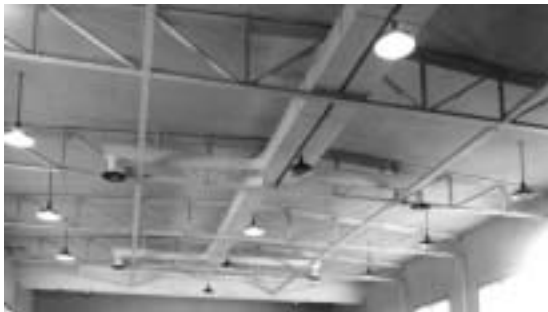
VIEW OF EXPOSED TRUSSES IN RECREATION ROOM LOOKING SOUTH (DETAIL BELOW). PHOTOGRAPH BY TERRY RISHEL (SEPTEMBER 2002).
